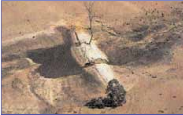
Small earth dam, broken due to lack of a sufficient spillway. Photo from booklet on water harvesting by the State Department in Western Australia.
