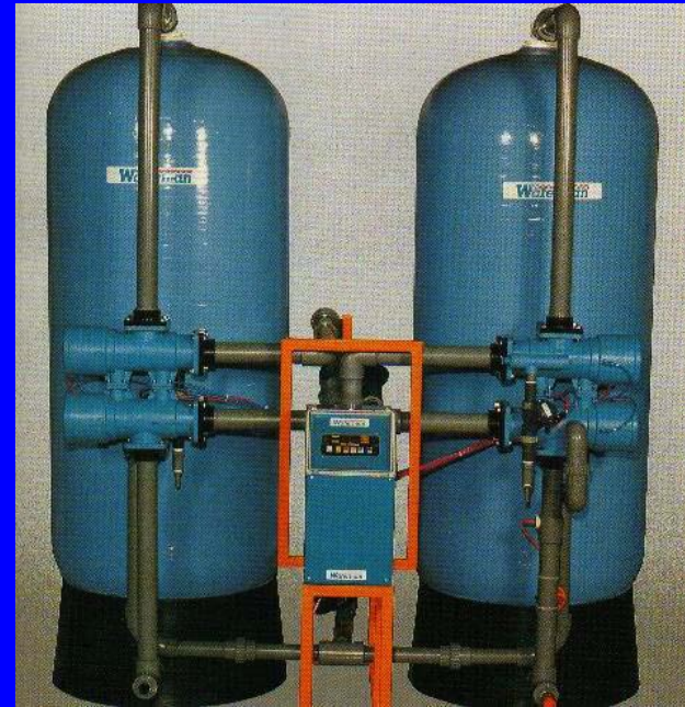
Ion exchange plant
