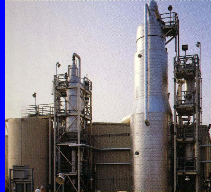
Evaporator - utility effluent
